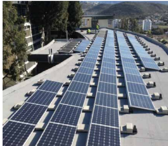
Figure 7: Ballast type mounting structure
